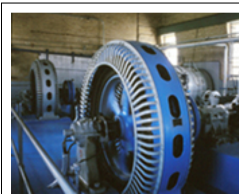
Utah Lake Pumping Plant Pump.
