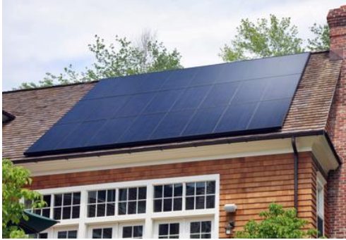
Figure 4. Roof-mounted solar panels
