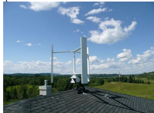
Figure 3. Roof-mounted wind energy system
