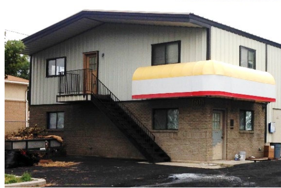
Figure 67 – Metal used is an industrial grade and has the appearance of standing seam metal which detracts from the architectural quality of the building.
