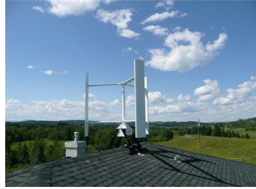
Figure 3. Roof-mounted wind energy system
