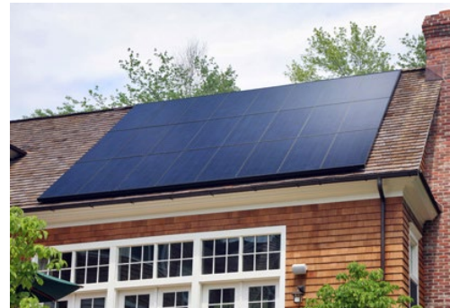
Figure 4. Roof-mounted solar panels
