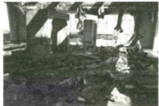
Figure 99 Cooling ponds after the fire
