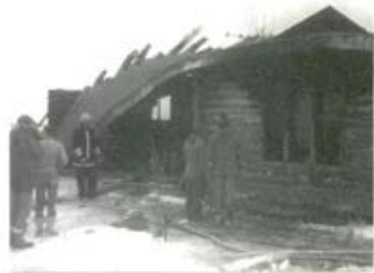
Figure 84 House fire in Fairfield
